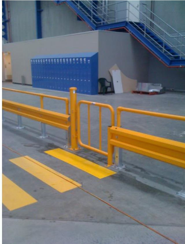
TRU-GARD™ Barrier, hand rail and personnel gates being installed at Manassen Foods in Sydney.
