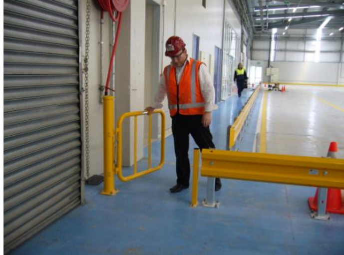
1 of 17 new TRU-GARD™ personnel gates being installed at the new Fonterra Distribution Centre in Dunedin.
