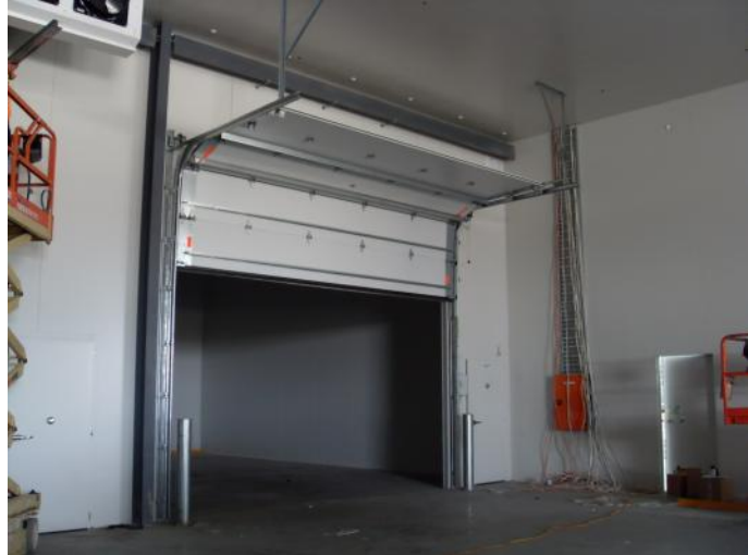
1 of 7 new TRU-THERM™ doors recently installed at the new DHL Distribution Centre in Melbourne.
