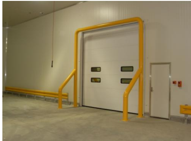
A newly installed TRU-SPRINT™ door in Ashburton, NZ being protected using TBI's TRU-GARD™ barrier and custom built door frame bollards.
