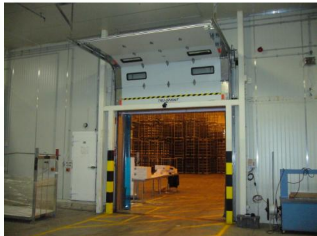
Silver Fern Farms—Silverstream Plant, Mosgiel, Dunedin NZ. — This TRU-SPRINT™ door was installed 2 years ago for product evaluation. This door operates at up to 250 cycles per day that's a whopping 182,000 cycles and still going strong.
